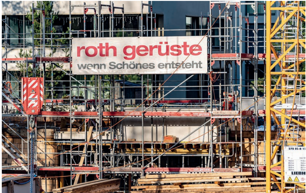
Scaffolding specialist Roth Gerüste at Seewarte's Park Schönbühl residential development in Zurich
